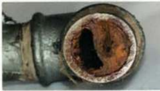
Pipe with scale deposits
